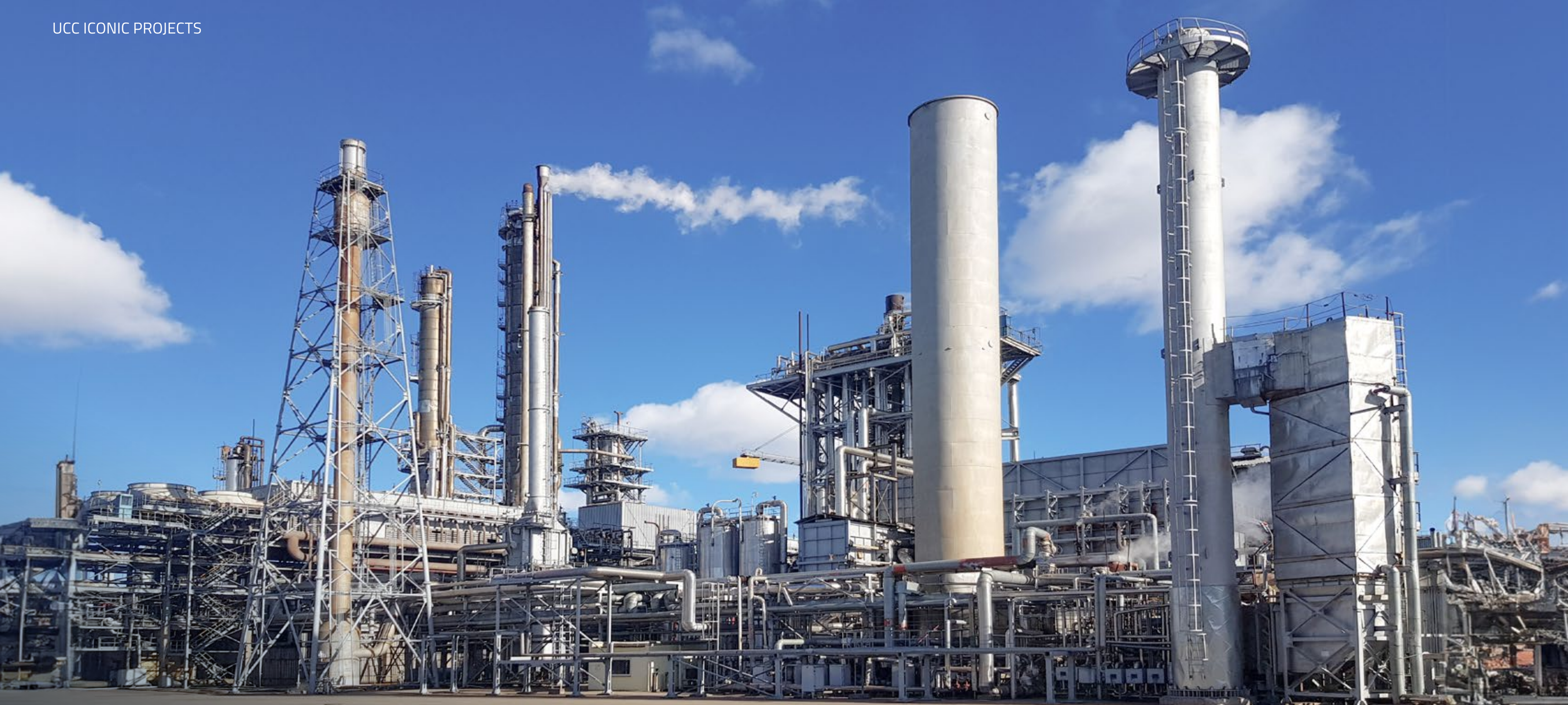
Petro Chemical Urea Ammonia Plant - Iraq
